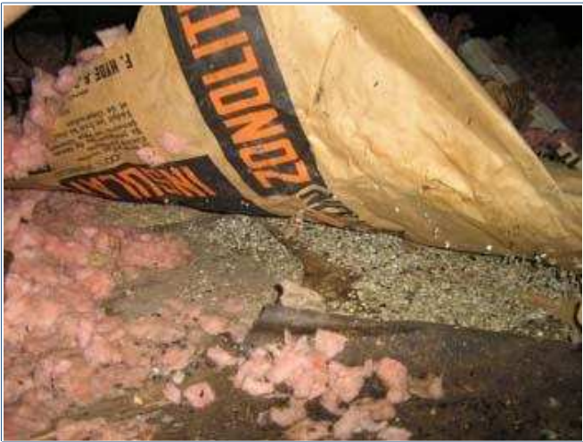
Suspect insulation: may contain asbestos
