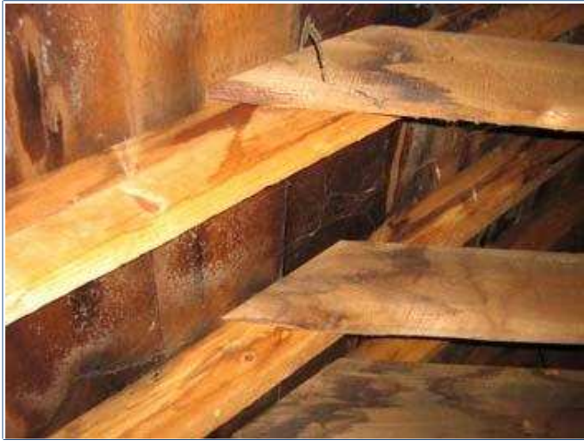
Water leak past roof cover and flashings, observed at attic
