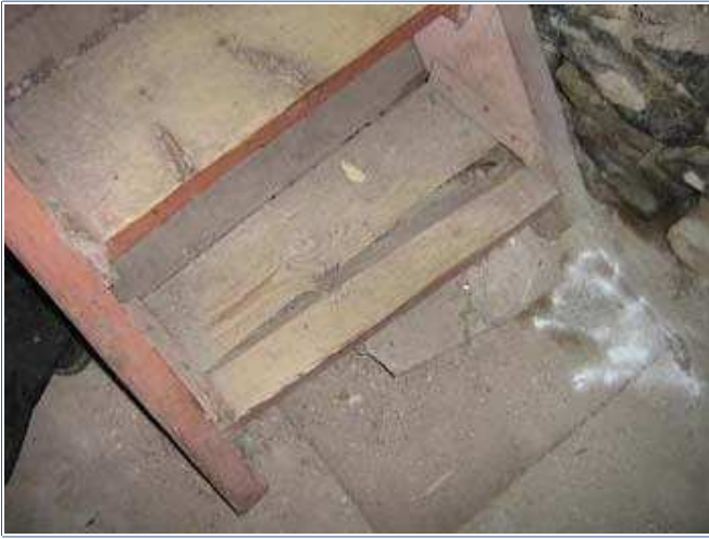
Damaged stair tread
