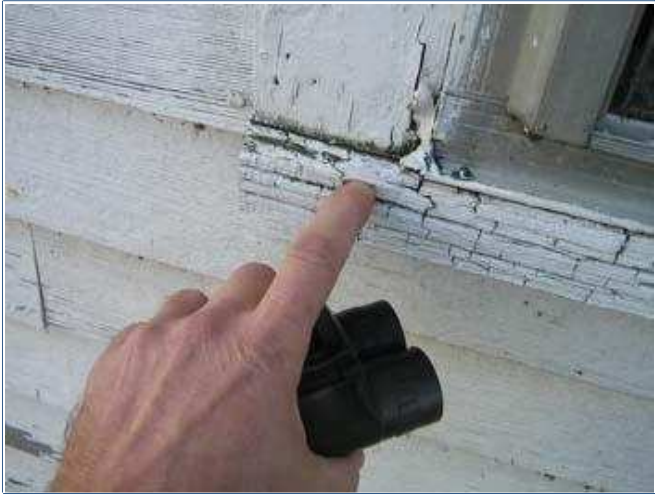
Deteriorated window frame; rot evident
