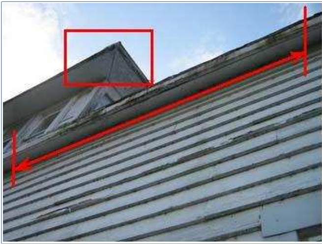
Deteriorated fascia; rot evident; secondary damage to soffits
