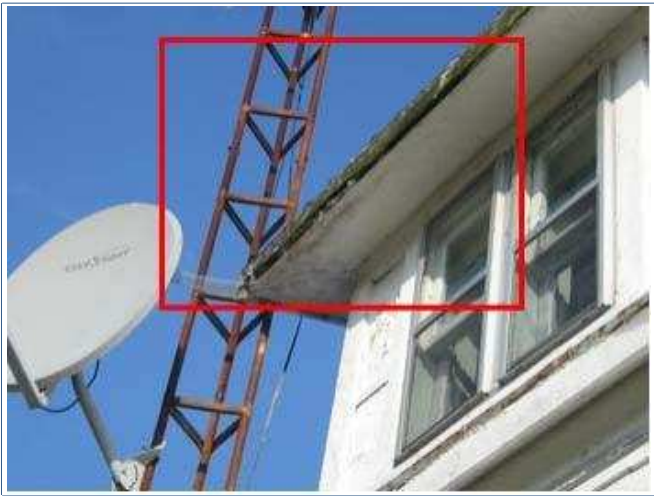
Deteriorated fascia; rot evident; leak past fascia damaging soffit.
