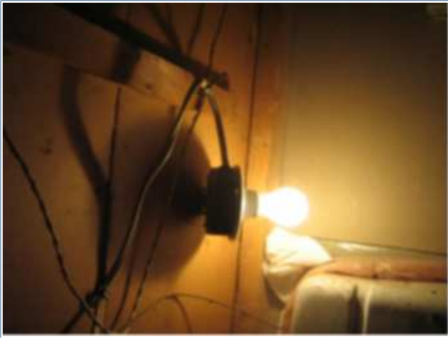
Light fixture improperly secured; near combustibles
