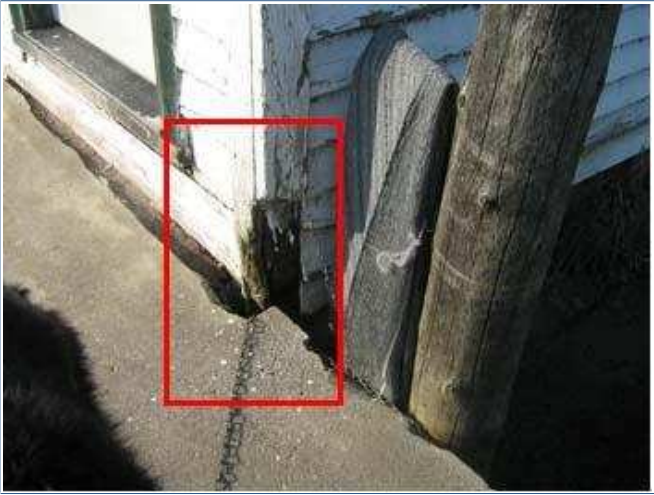
Deteriorated wood near grade level; rot evident
