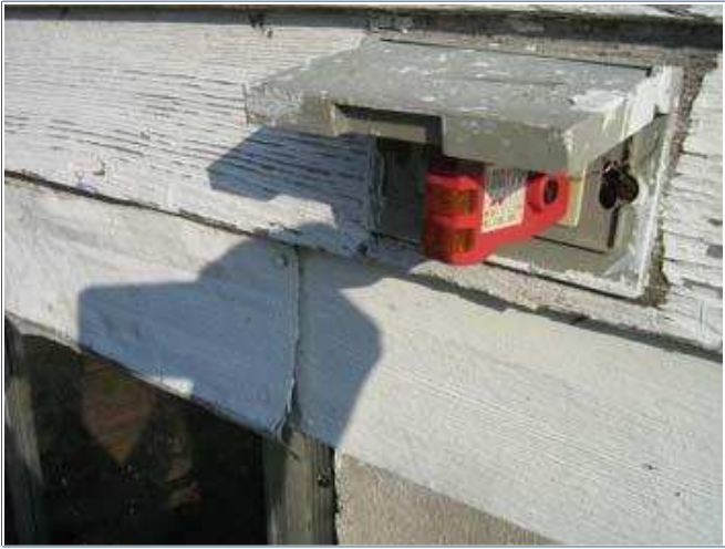
Defective outlet: fails to reset
