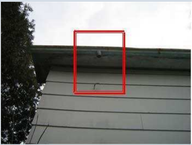
Missing downspout from gutter
