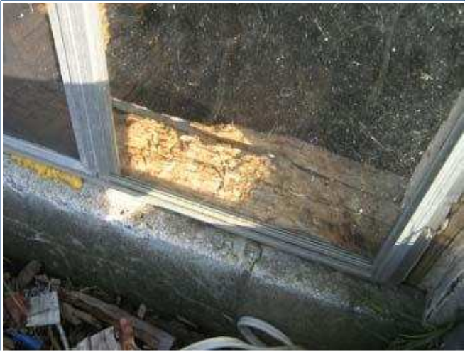
Deteriorated window frame; dry and wet rot evident
