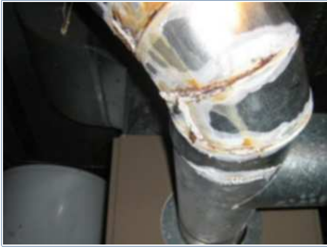
Corrosion in furnace exhaust ducting
