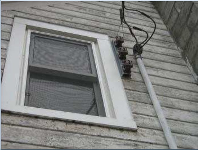
Electrical mast & weatherhead near openable window
