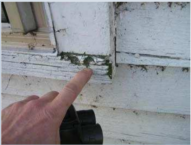
Deteriorated window frame; rot evident
