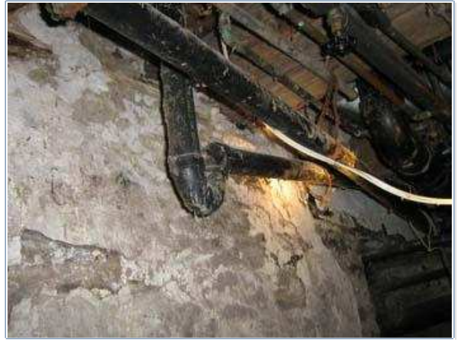
Improper slope, drainage pipe
