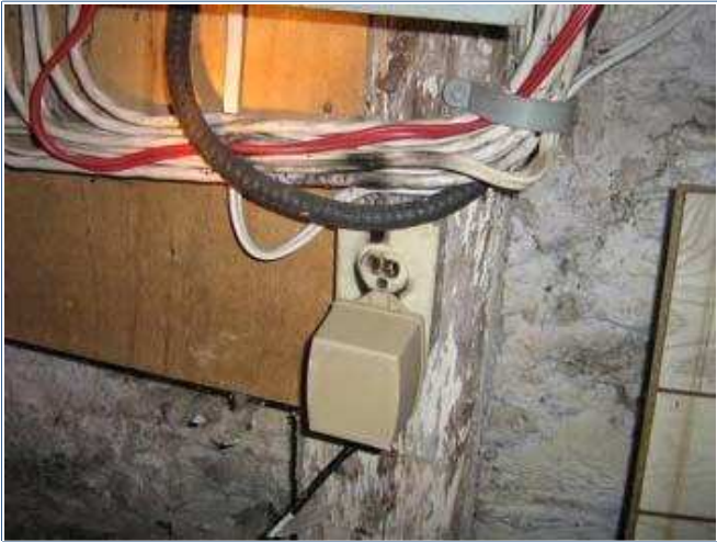
Charred electrical wiring
