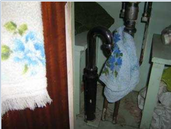
S-trap below sink
