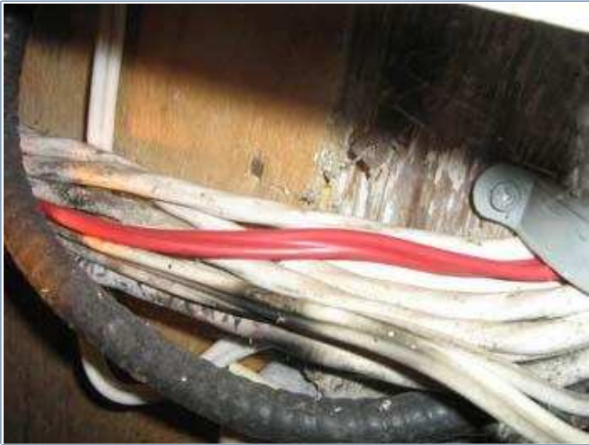
Charred electrical wiring near main electrical panel
