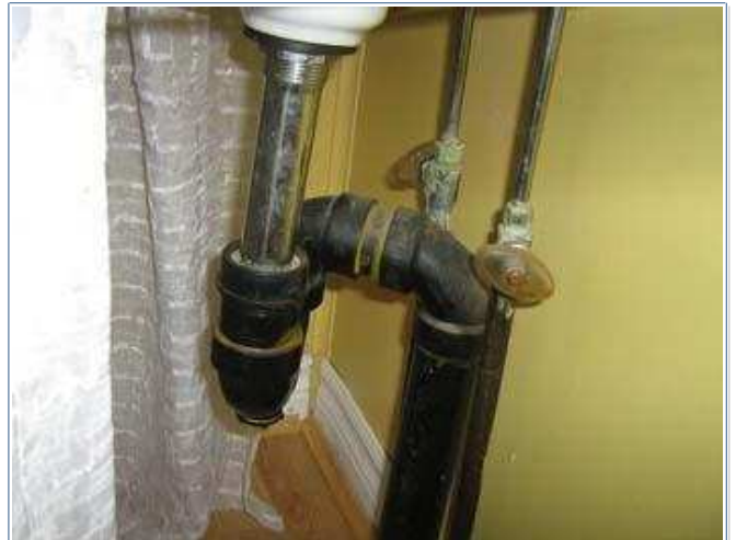
S-trap below sink
