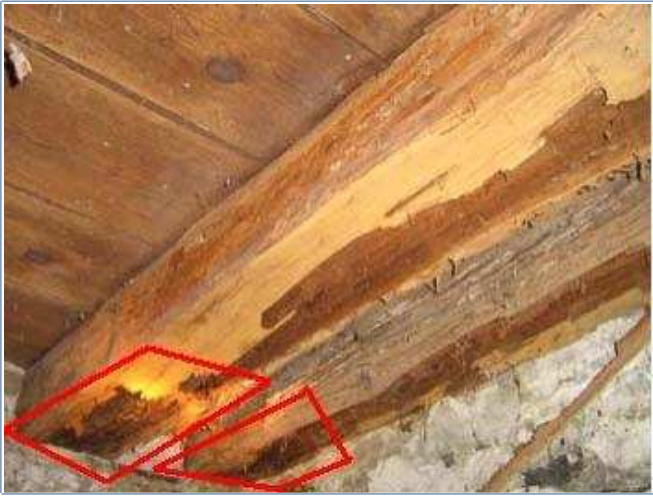
Rooted beam at pocket; dry and wet rot observed
