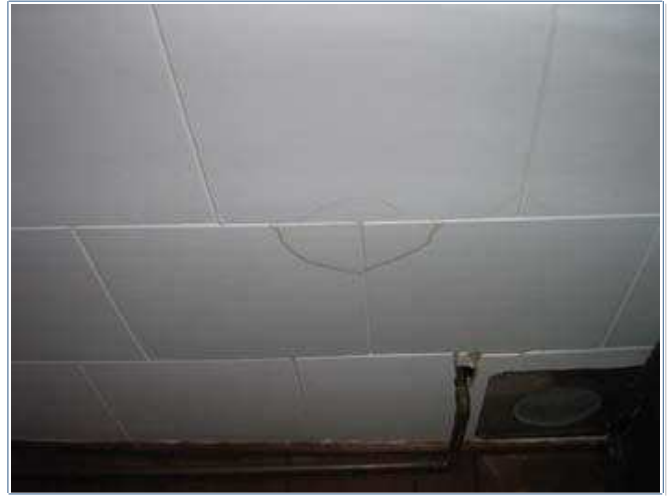
Water staining on ceiling tiles
