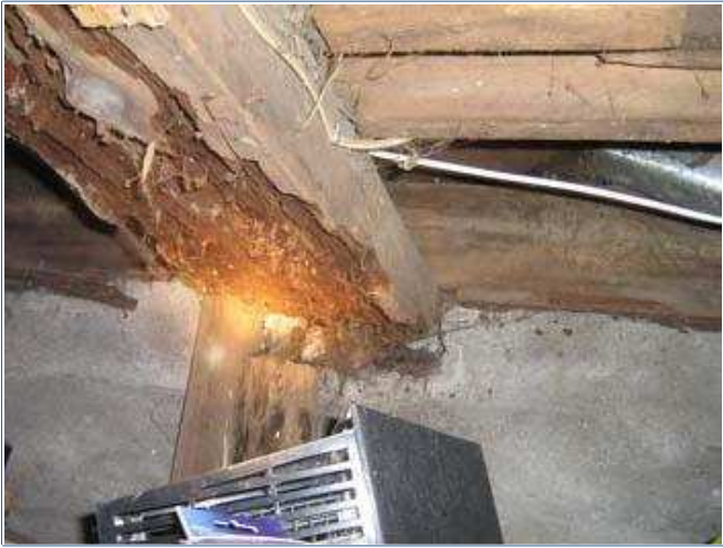
Rotted beam in basement; dry rot suspected
