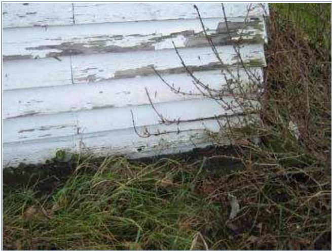
Deteriorated wood near grade level; rot evident
