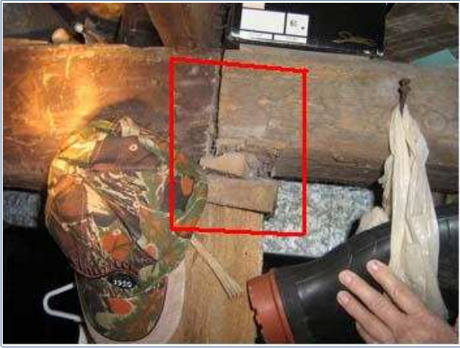
Improper beam bearing; improper column end bearing
