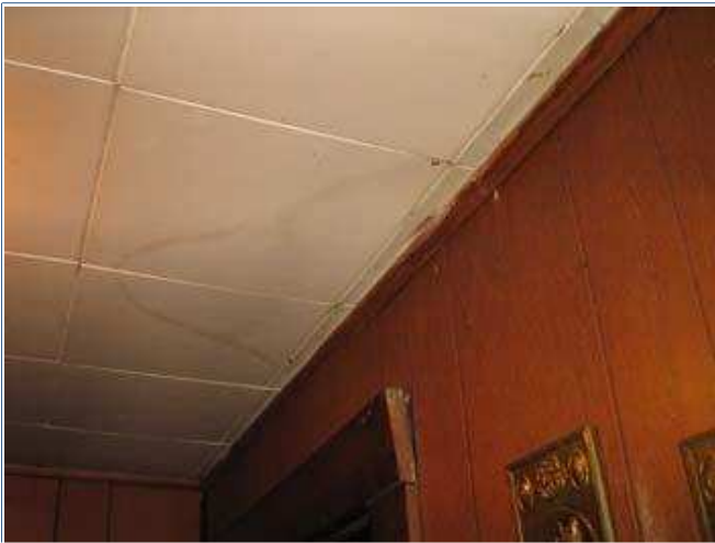
Water staining on ceiling tiles
