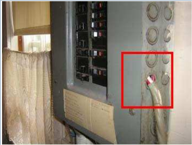
Missing wire protection at main electrical panel
