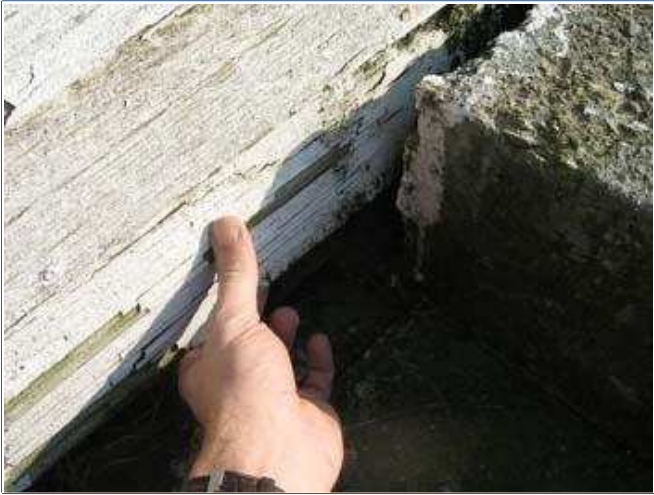
Deteriorated wood siding near grade; rot evident
