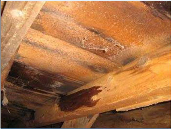
Leak past roof cover as viewed from attic
